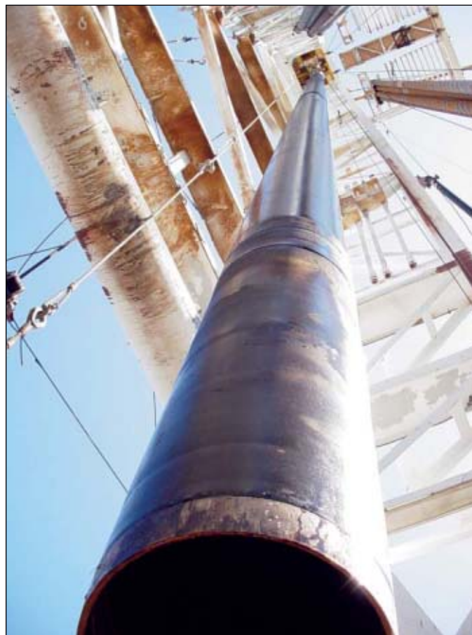
After expansion, the monobore liner extension system is pulled from the test well (Fig. 3).
